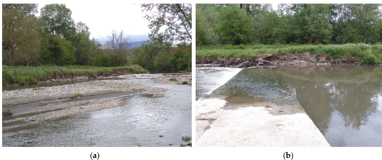
Figure 5. Field images illustrating indirect evidence of riverbed lowering due to channel incision: (a) ~1 m-high fluvial erosional scarp; (b) fluvial erosional scarp and weir deformed by undermining processes connected to riverbed degradation.
