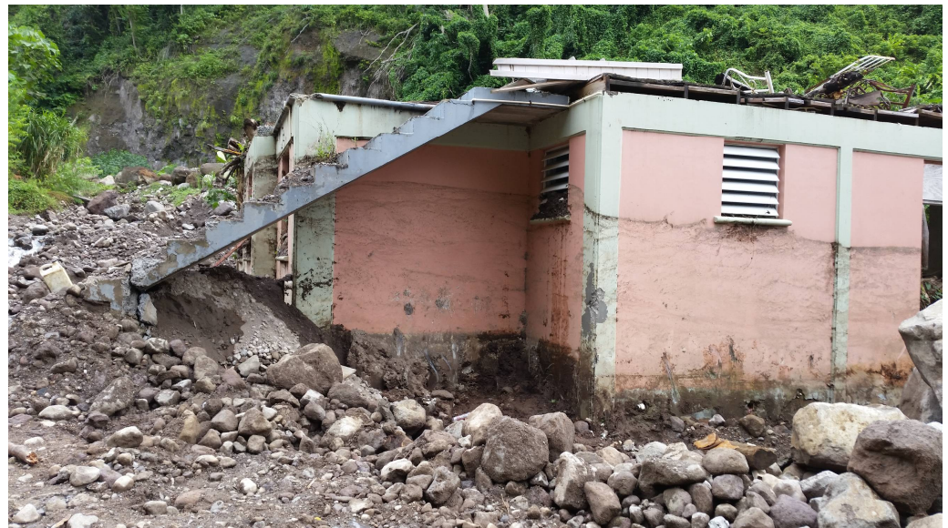
Figure 1. Debris and sediment deposition around a building in Castle Comfort, Dominica, following extreme rainfall during Hurricane Maria.
