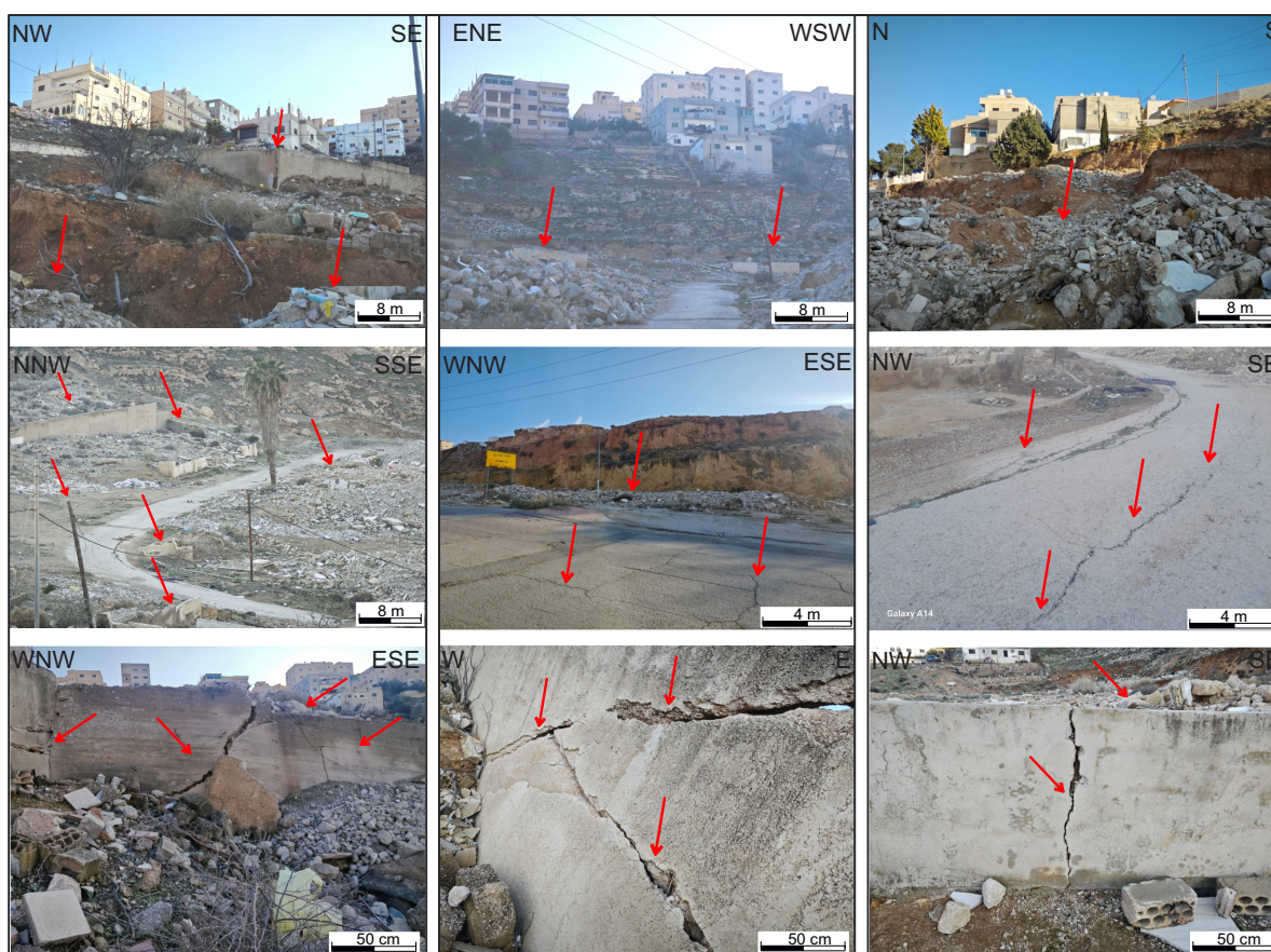
Figure 14. Photographs of landslides triggered by recent fault activity in the northwestern extension of the KWF. Red arrows indicate landslide expression.
