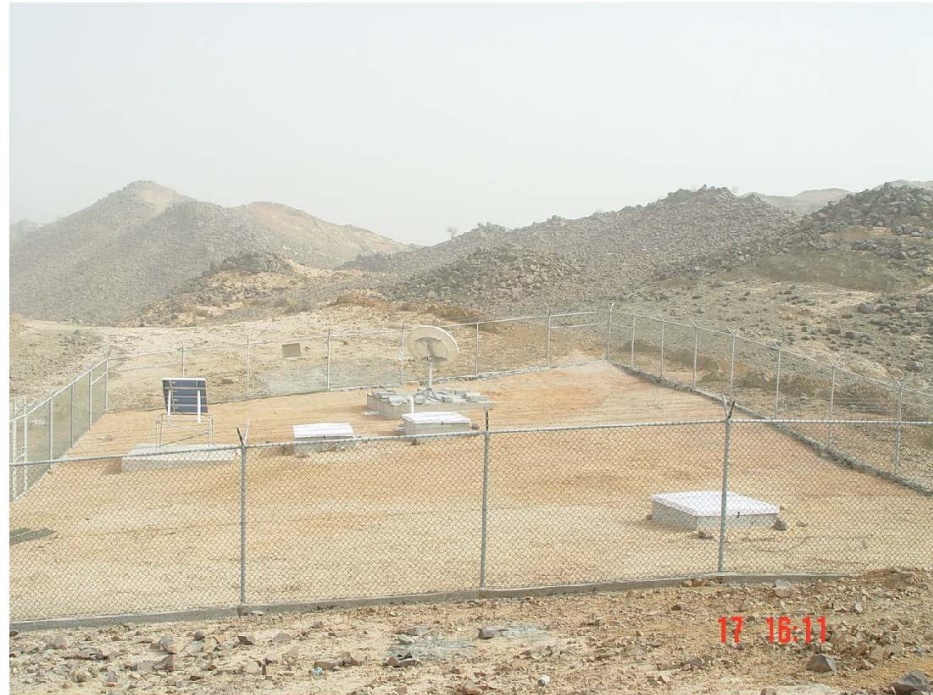
Figure 2. The installation of SNSN station number 9, located in the Arabian Shield area. Each station consists of Nanometrics Trillium 40 seismometers, 24-bit Trident digitizers, GPS receivers, and Cygnus VSAT transceivers and powered by a 320-watt solar array.
