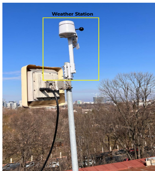
Figure 7. The weather station is used to take in outdoor data.
