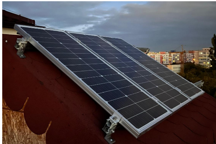
Figure 2. Photovoltaic Panels Used in the Developed System.
