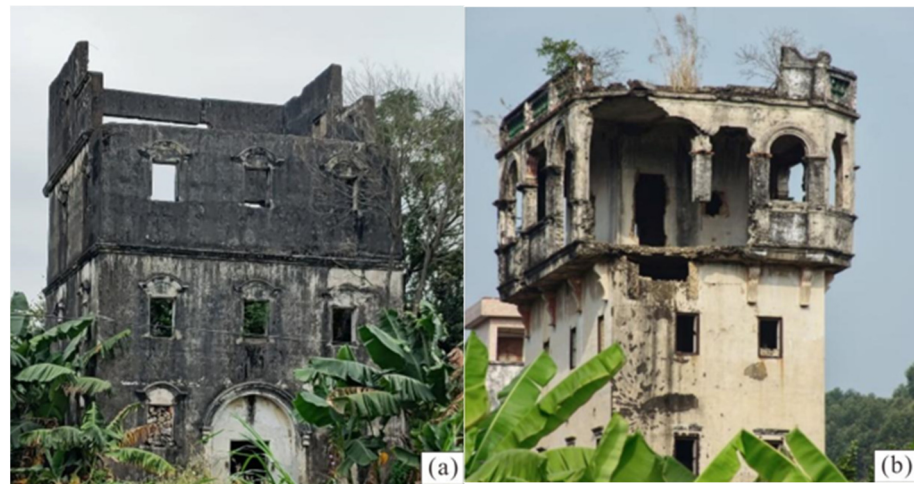
Figure 5. Damaged architectural cultural heritage of Kaiping Diaolou. (a) Diaolou 1; (b) Diaolou 2. Photographed by Le Gao in Kaiping, Jiangmen, China, in July 2025.
