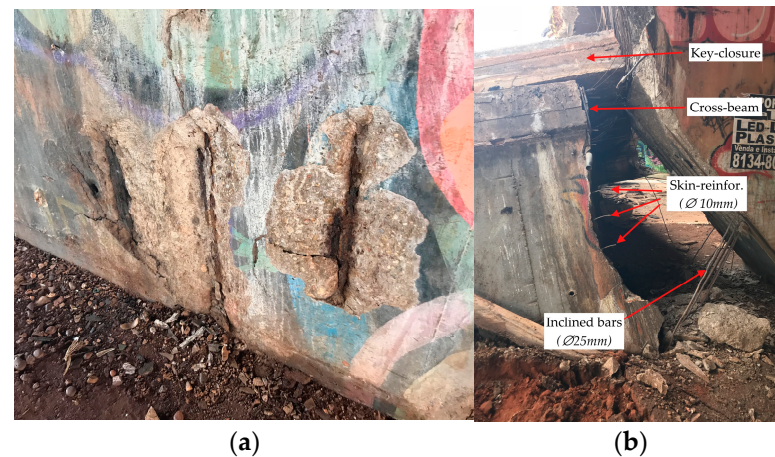
Figure 11. Investigation of debris: (a) severe corrosion of column rebars near ground level; (b) fallen section, indicating cut rebars and inclined column bars that had peeled out.
