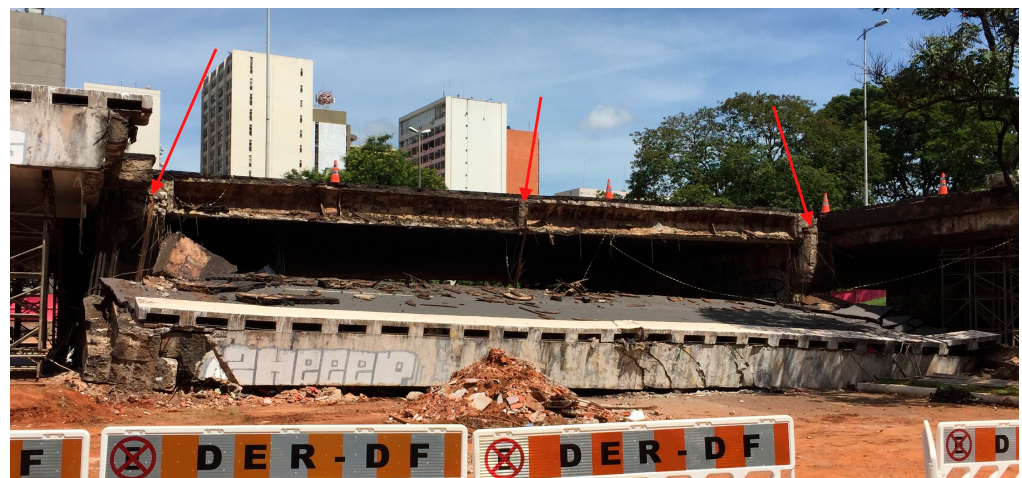
Figure 1. Section of the viaduct at Galeria dos Estados after the partial collapse in 2018, with indication of fracture of the main elements.
