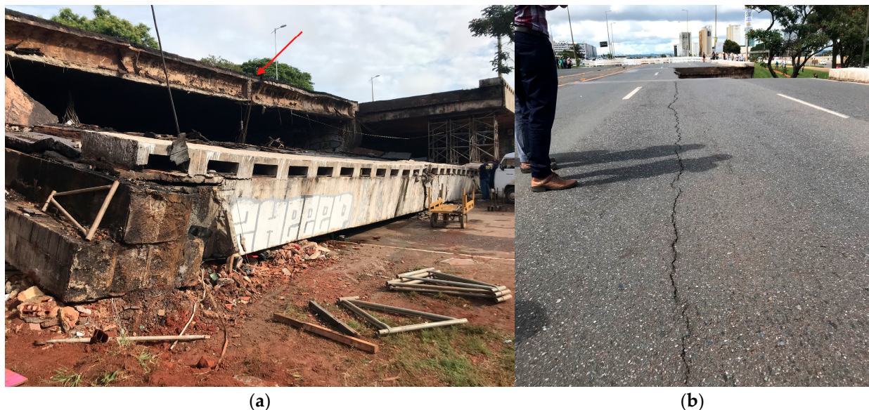
Figure 8. Investigation of the debris: (a) section of the deck that collapsed, highlighting the transverse beam that failed under shear (indicated by the red arrow); (b) large longitudinal asphalt crack across the deck next to the fallen section between column walls P5 and P6.
