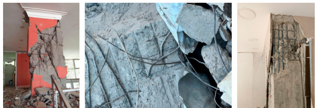
Figure 11. Insufficient concrete-reinforcement interlock resulting from the use of plain reinforcement.
