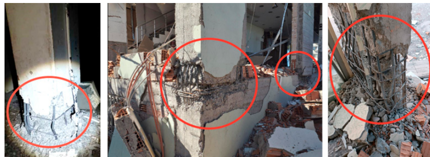
Figure 7. Examples of failures in the lower end of the column.
