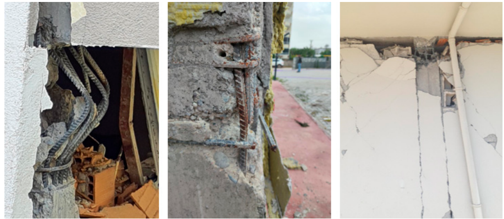
Figure 12. Buckling samples in longitudinal reinforcement.
