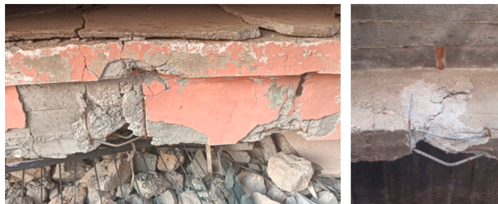
Figure 24. Lateral buckling failure in RC beams.
