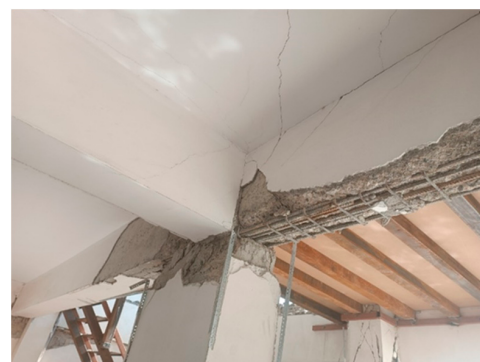
Figure 22. Insufficient concrete cover thickness in the RC beam.
