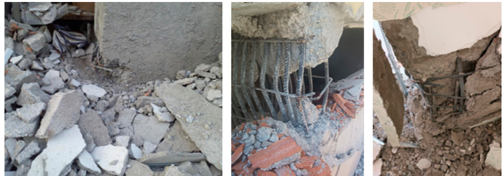
Figure 17. Examples of slips of transverse reinforcement caused by insufficient anchorage of 90^\circ hooks during earthquake loading.
