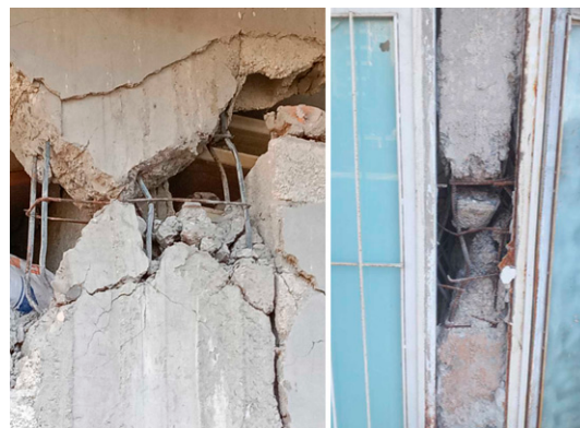
Figure 8. Failures in the middle region of the column.
