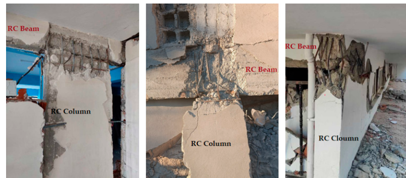
Figure 5. Illustrations of structural failure modes, characterized by the simultaneous crushing of the concrete matrix and lateral buckling of longitudinal bars due to inadequate stirrup configurations in beam-column joints.
