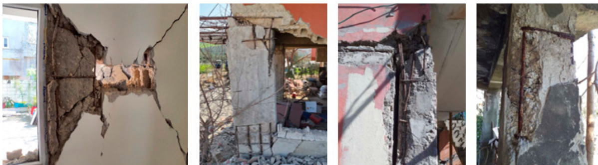
Figure 14. Examples of failure from insufficient transverse reinforcement and concrete cover.
