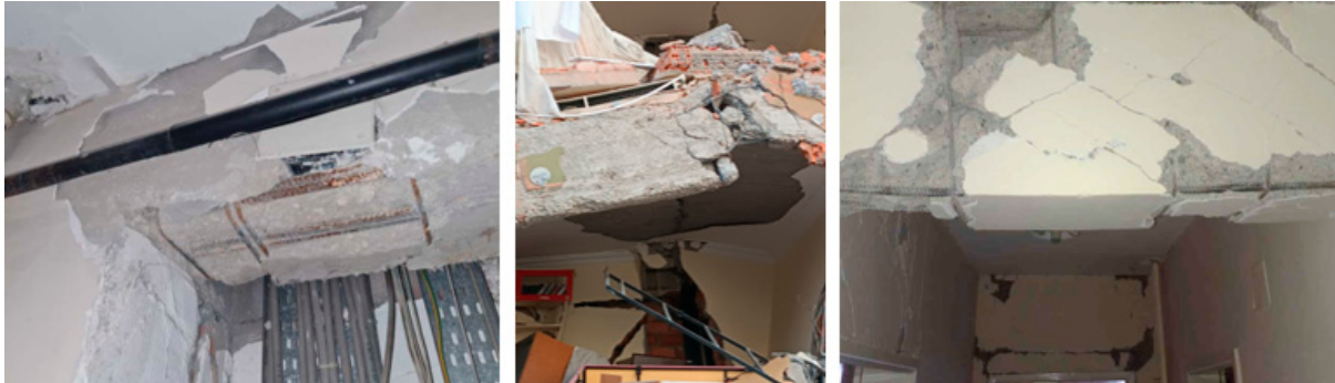
Figure 23. Examples of failure caused by insufficient transverse reinforcement in beams.
