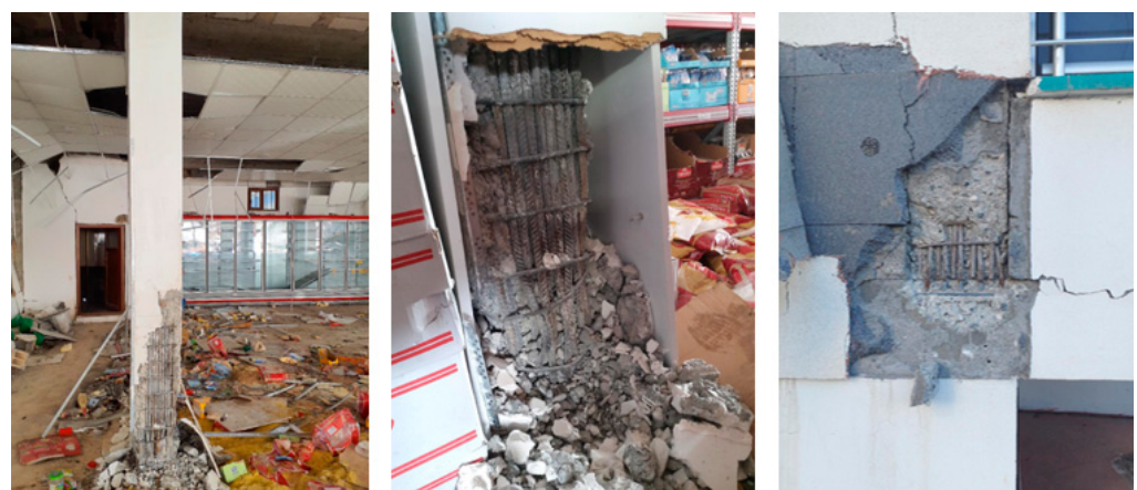
Figure 9. Examples of failures resulting from the failure of transverse reinforcements to perform their expected functions due to excessive use of longitudinal reinforcement.
