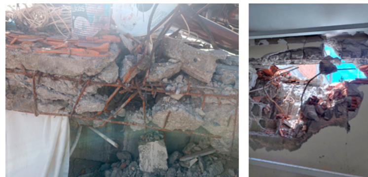
Figure 25. Examples of failure caused by corroded plain reinforcement.
