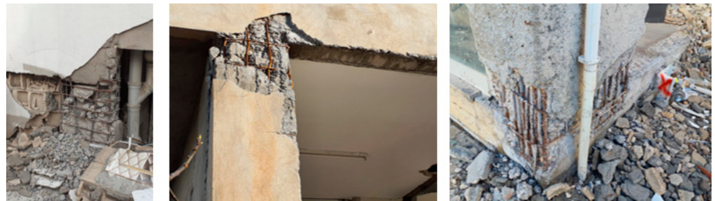
Figure 13. Corroded reinforcement and insufficient interlock resulting from inadequate concrete cover thickness.
