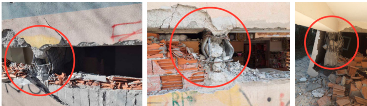
Figure 10. Buckling of longitudinal reinforcement due to insufficient transverse reinforcement in short columns.
