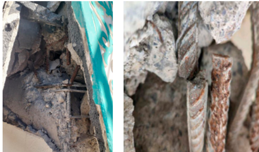
Figure 15. Fracture in the longitudinal reinforcement.
