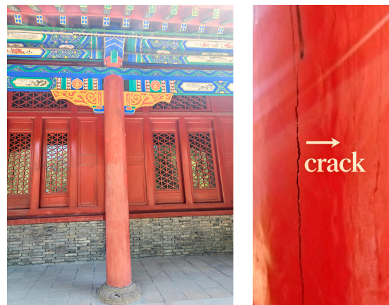
Figure 4. Current condition of load-bearing timber columns in the Bawang Academy Ancient Timber Structures.
