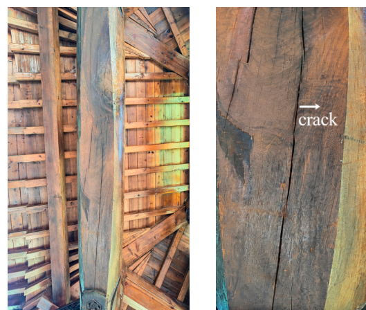
Figure 5. Current condition of load-bearing timber beams in the Bawang Academy ancient timber structures.
