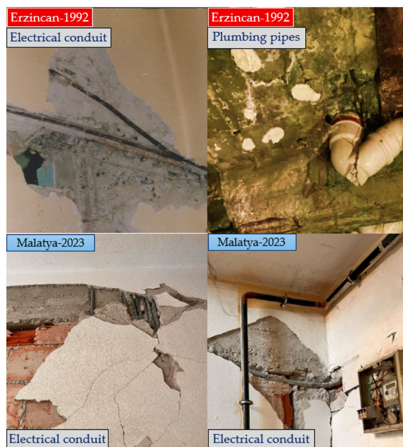
Figure 7. User-related construction mistakes involving electrical conduits and water pipes embedded in reinforced concrete members observed in the 1992 Erzincan and 2023 Malatya earthquakes.
