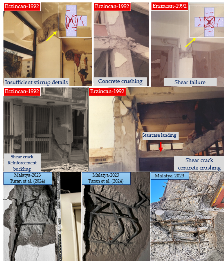
Figure 13. Column–beam joint damage and shear failure patterns observed in reinforced concrete buildings following the 1992 Erzincan and 2023 Malatya earthquakes, including insufficient stirrup detailing, concrete crushing, shear cracking, and reinforcement buckling. The Malatya-2023 observations are based on field data reported in Turan et al. (2024) [43].
