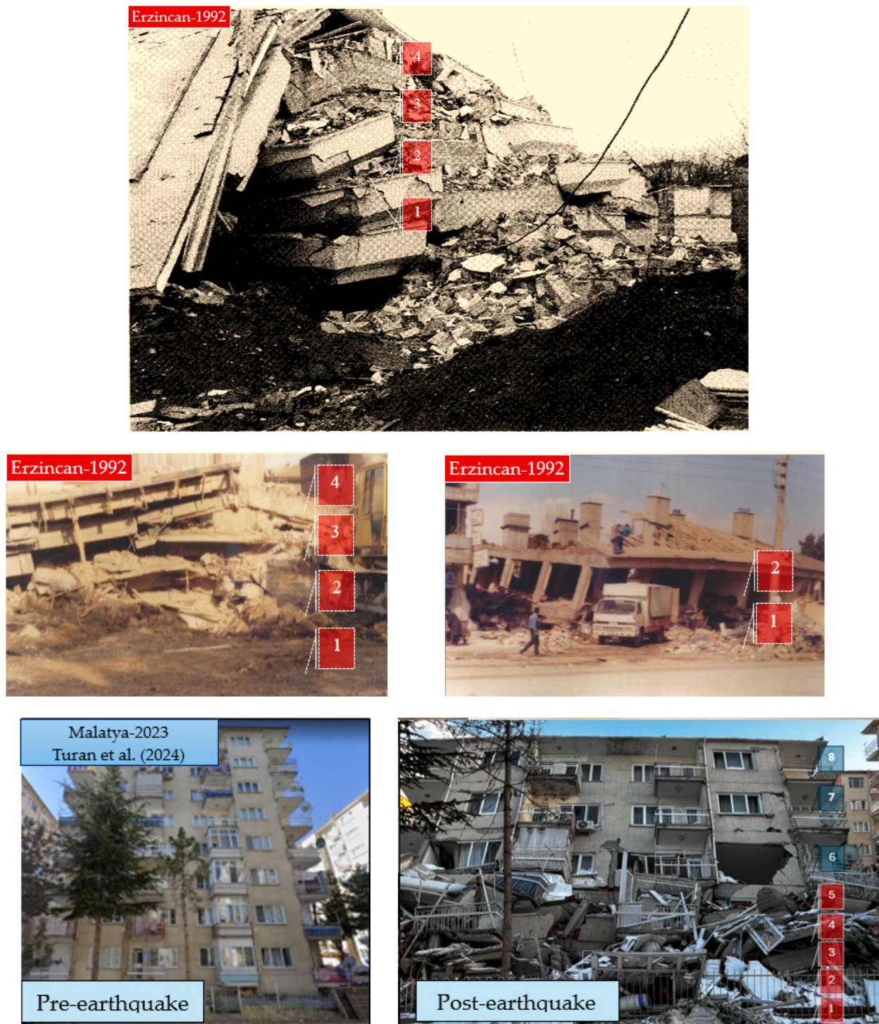
Figure 24. Examples of progressive collapse observed in multi-story reinforced concrete buildings in Erzincan (1992) and Malatya (2023): the sequential failure of lower-story columns led to upper-story collapse, highlighting weak-story mechanisms and stiffness irregularities. Numbered annotations indicate the sequence of failure across stories. The Malatya-2023 case is based on field observations reported in Turan et al. (2024) [43], with additional visual representation for comparative documentation purposes.
