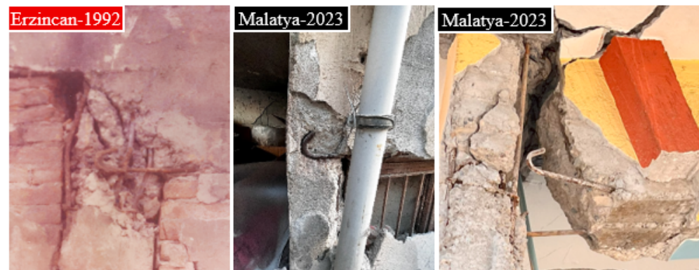
Figure 19. Examples of inadequate hook detailing and insufficient anchorage observed in reinforced concrete members following the 1992 Erzincan and 2023 Malatya earthquakes.
