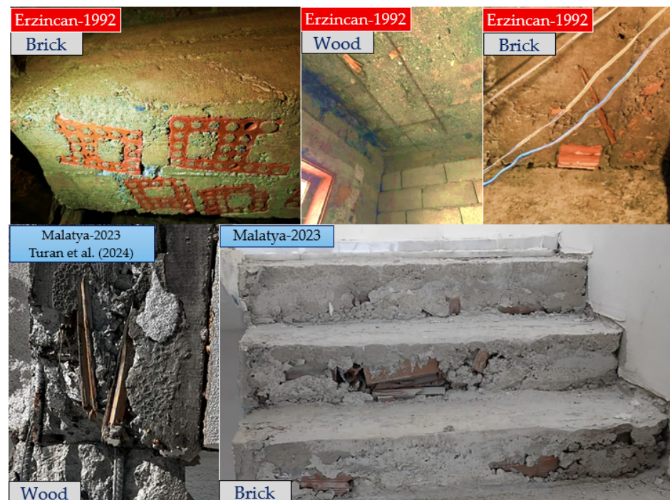
Figure 6. Examples of foreign materials embedded in concrete observed in reinforced concrete buildings following the 1992 Erzincan and 2023 Malatya earthquakes, including brick and wood inclusions. The Malatya-2023 case is based on field observations reported in Turan et al. (2024) [43], with additional visual representation for comparative documentation purposes.
