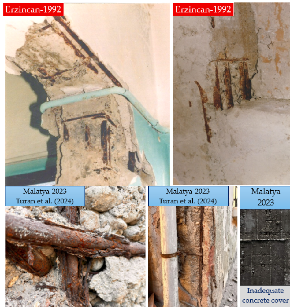
Figure 8. Examples of corrosion-induced deterioration and inadequate concrete cover observed in reinforced concrete members following the 1992 Erzincan and 2023 Malatya earthquakes. The Malatya-2023 case is based on field observations reported in Turan et al. (2024) [43], with additional visual representation for comparative documentation purposes.
