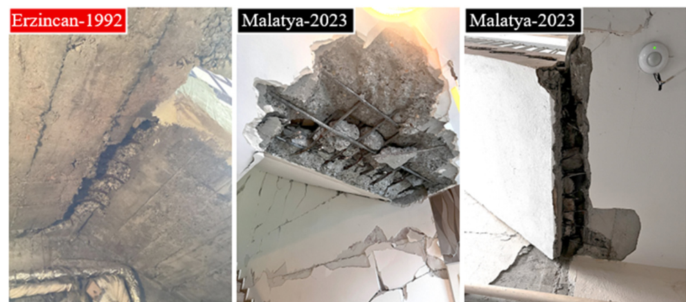
Figure 28. Examples of cracking and local crushing damage observed in reinforced concrete staircase landing regions following the Erzincan (1992) and Malatya (2023) earthquakes.
