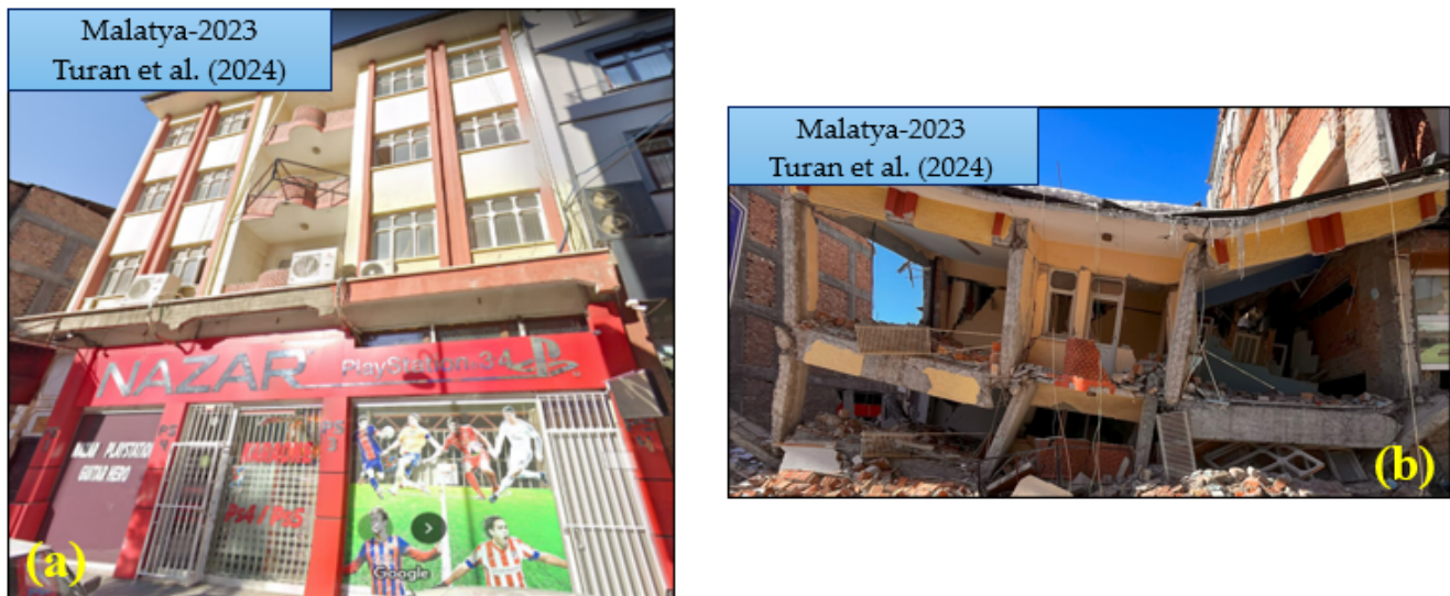
Figure 16. (a) Pre-earthquake and (b) post-earthquake views of a reinforced concrete building in Malatya Province exhibiting severe soft-story collapse behavior following the 2023 Kahramanmaraş earthquake sequence. The Malatya-2023 case is based on field observations reported in Turan et al. (2024) [43], with additional visual representation for comparative documentation purposes.
