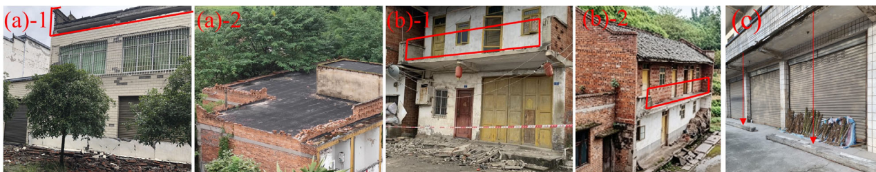
Figure 12. Accessory components damage. (a)-1, (a)-2 Parapet wall collapse. (b)-1, (b)-2 Railing collapse. (c) Walkway precast slab falling.
