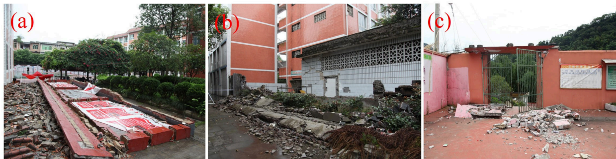
Figure 15. Typical independent structural seismic damage. (a) School display wall collapse. (b) Perimeter wall collapse. (c) Plaque collapse on a wall.
