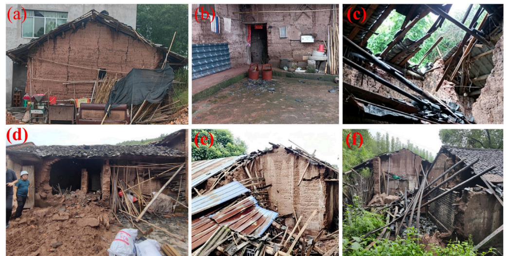
Figure 14. Typical seismic damage to earthen structures. (a) Widening of pre-existing cracks. (b) Slipped roof tiles. (c) Failure of wooden roof truss. (d) Local collapse of wall. (e) Complete collapse. (f) Complete collapse.
