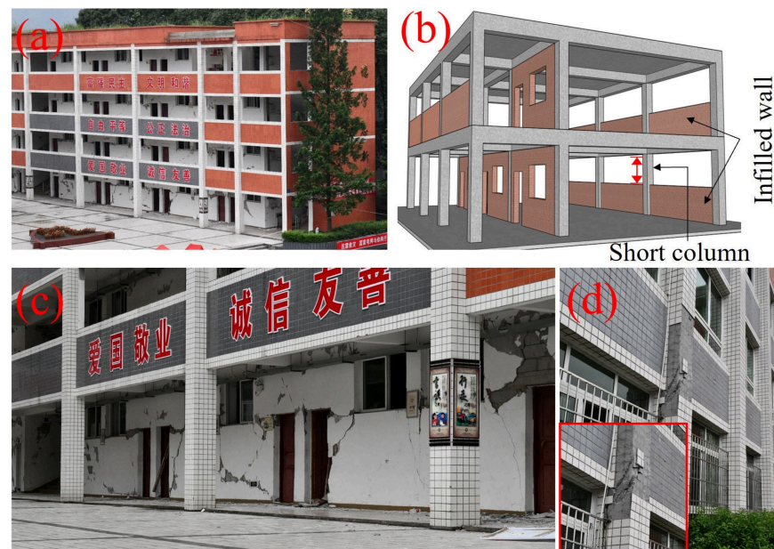
Figure 6. Construction forms and damage characteristics of a typical frame structure. (a) Overall exterior view of the building. (b) Schematic layout of internal longitudinal beams, columns, and walls. (c) Infill wall damage on the front elevation. (d) Column shear failure on the rear elevation.
