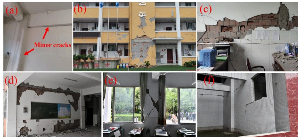
Figure 7. Failure modes of infill walls. (a) Minor cracks at wall-frame interface. (b) Internal cracks in infill wall. (c) Damage of infill wall with porous shale bricks. (d) Damage of infill wall with solid bricks. (e) Short column failure. (f) Cracks at wall-frame interface in shear wall structure.
