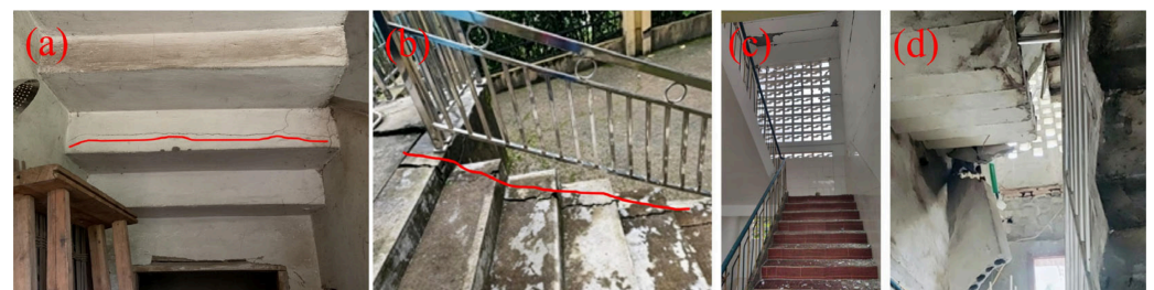
Figure 10. Typical seismic damage to staircases. (a) Transverse cracks on stair flight. (b) Longitudinal cracks on stair flight. (c) Wall damage in staircase. (d) Stair flight collapse.
