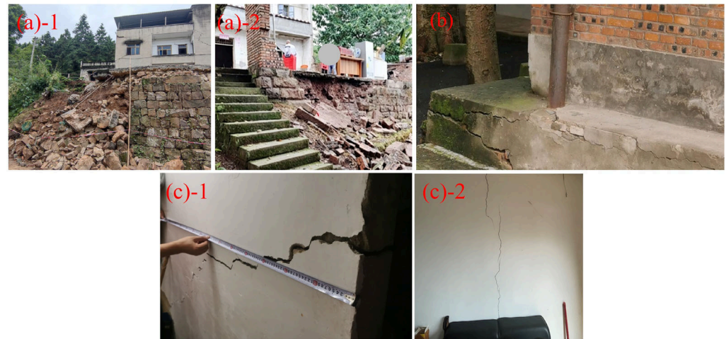
Figure 11. Seismic damage to foundations and substructures. (a)-1, (a)-2 Damage to foundation maintenance structure. (b) Foundation damage. (c)-1, (c)-2 Wall cracks caused by uneven settlement of the foundation.
