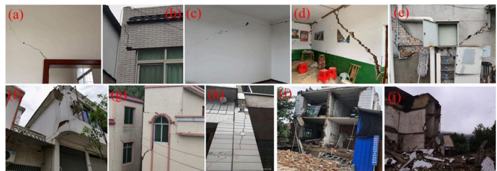
Figure 8. Failure modes of load-bearing walls. (a) Diagonal cracks at door opening. (b) Diagonal cracks at window opening. (c) Minor diagonal cracks. (d) Severe diagonal cracks. (e) Cross cracks; (f) Corner cracks. (g) Attic cracks. (h) Collision cracks. (i) Collapse of front longitudinal wall. (j) Complete collapse.
