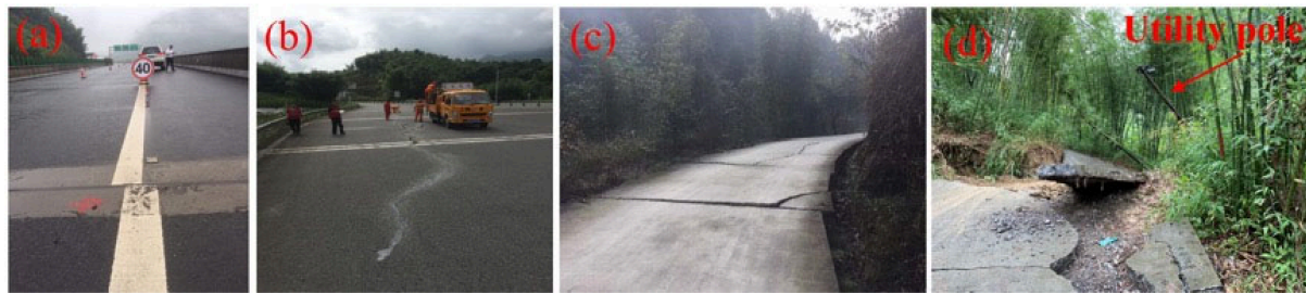
Figure 17. Earthquake damage to roads and power lines. (a) Bridge displacement. (b) Cracks in urban asphalt pavement. (c) Cracks in rural concrete pavement. (d) Damage to roads and power transmission lines.
