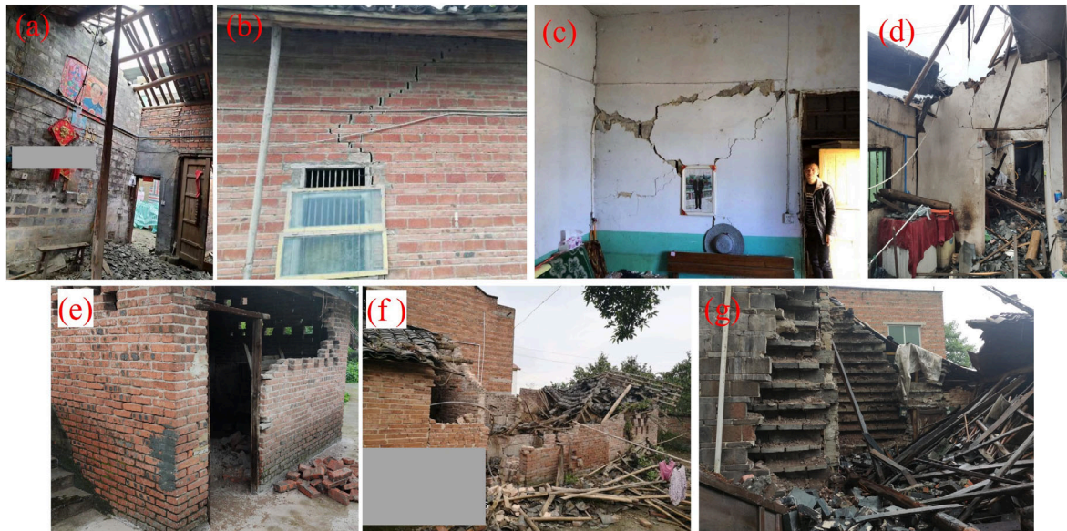
Figure 13. Typical seismic damage to brick-timber structures. (a) Slipped roof tiles. (b) Stepped cracking. (c) Failure of load-bearing wall. (d) Collapse of wooden roof. (e) Local spalling of wall. (f) Complete collapse of building. (g) Failure of cavity wall.
