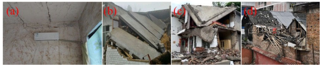
Figure 9. Typical seismic damage to floors and roofs. (a) Cracking in precast floor slabs. (b) Collapse of precast floor slabs. (c) Local collapse of cast-in-place floor slabs. (d) Collapse of wooden roof truss.
