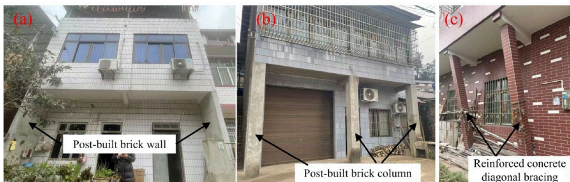
Figure 25. Current self-designed reinforcement measures by residents. (a) Later-added brick wall. (b) Later-added brick column. (c) Additional reinforced concrete diagonal bracing.
