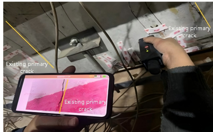
Figure 8. Record of crack parameters in T-beams.
