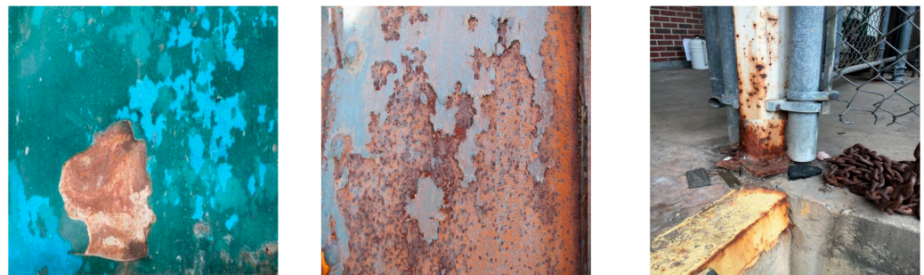
Figure 1. Corrosion characteristics of steel structures.
