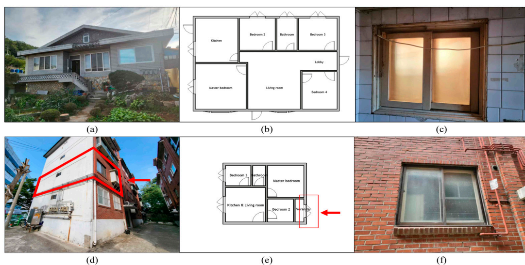
Figure 1. Examples of detached and multi-family houses for window retrofits. (a–c) Detached house: exterior view, simplified floor plan indicating window locations, and close-up photos showing deteriorated aluminum frames and condensation traces. (d–f) Multi-family house: exterior view, floor plan, and close-up views of aged single-glazed windows with poor sealing.
