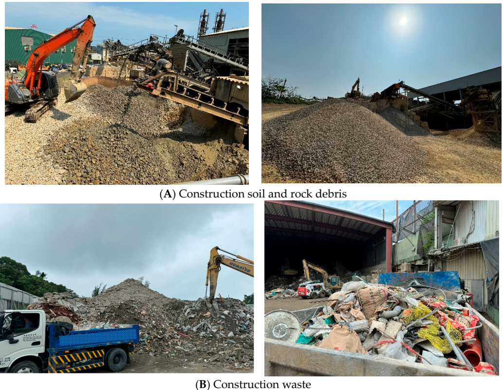
Figure 3. Photograph of construction soil and rock debris, and construction waste (photos were shot by the authors).
