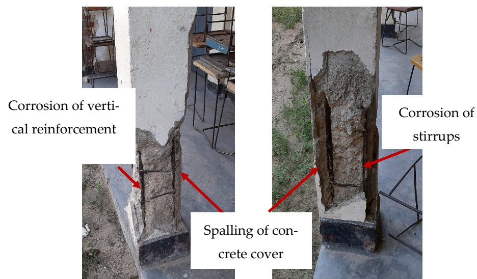
Figure 1. Corrosions noticed in RC columns.
