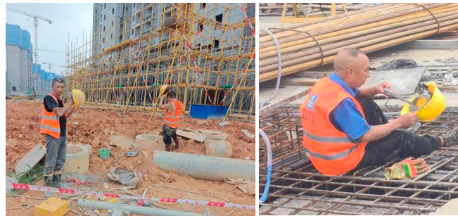
Figure 1. Workers on construction sites without helmets.
