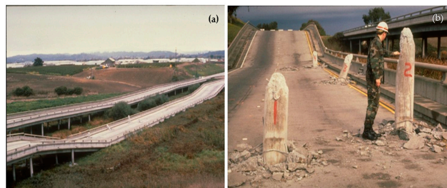
Figure 7. Vertical earthquake-induced phenomena at Struve Slough bridge in the Loma Prieta earthquake: (a) Collapse of bridge at Struve Slough [108]; (b) Detail of punching failure [109].
