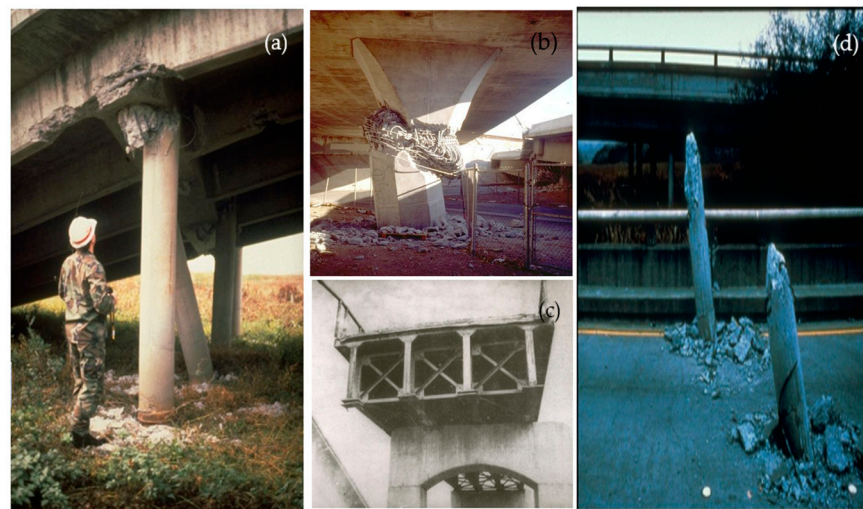
Figure 8. Seismic damage of bridge piers due to vertical seismic excitation (a) Vertical pounding-induced eccentric collisions [118]; (b) axial crushing of piers [119]; (c) unseating failures resulting from degraded girder–bearing contact [120]; (d) upper pier and girder damage triggered by vertical seismic pounding [118].
