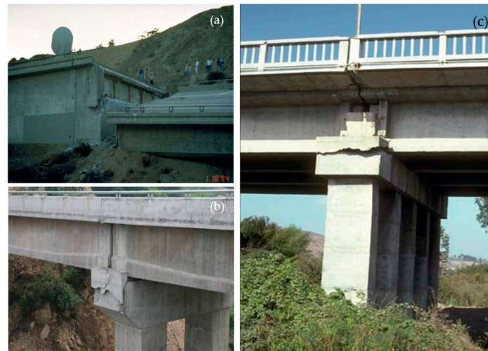
Figure 3. Various shear key seismic failures (a) Northridge Earthquake [33]; (b) Wenchuan Earthquake [28]; (c) Chile Earthquake [34].
