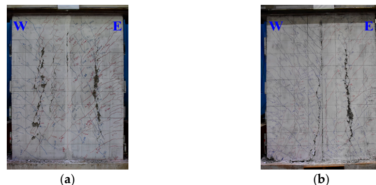
Figure 7. Failure mode of specimens at ultimate point. (a) PSW1-A. (b) PSW1-B.
