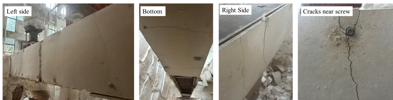
Figure 16. Cracks and peeling of the fiber cement board.
