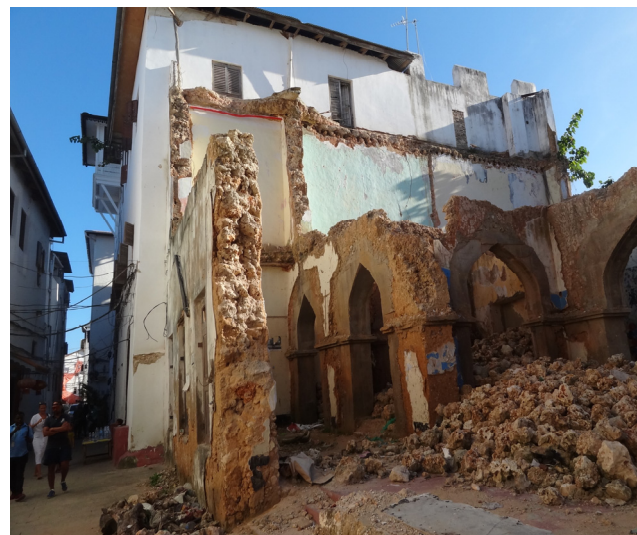
Figure 4. Example of the collapsed building (photos by author).
