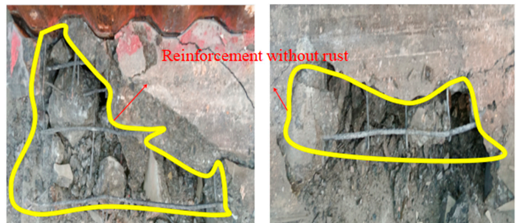
Figure 8. Corrosion of reinforcement.
