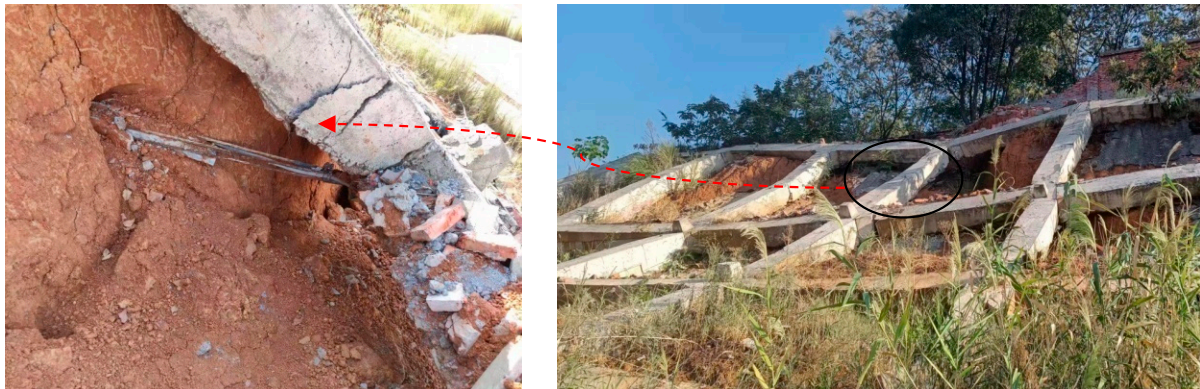
Figure 2. A case of structural damage of lattice beam.
