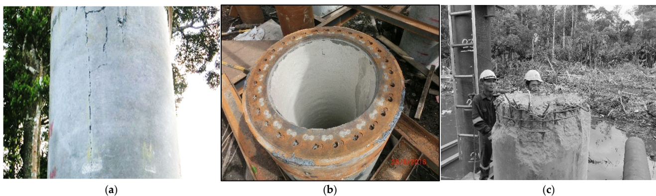
Figure 6. Failure types of the PHC pipe pile driving. (a) Pile shaft breakage; (b) Weld tearing; (c) Pile head breakage.
