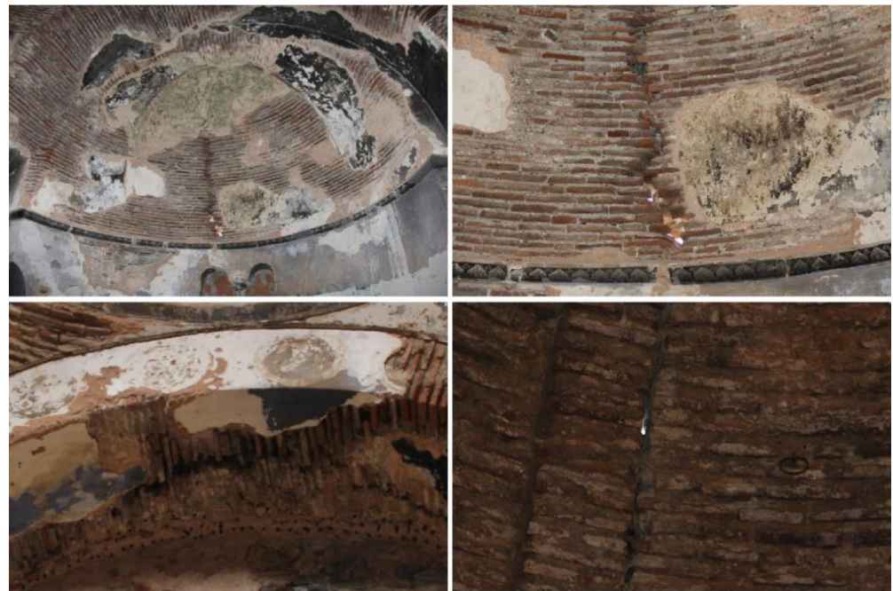
Figure 7. Cracks in the domes and arches.
