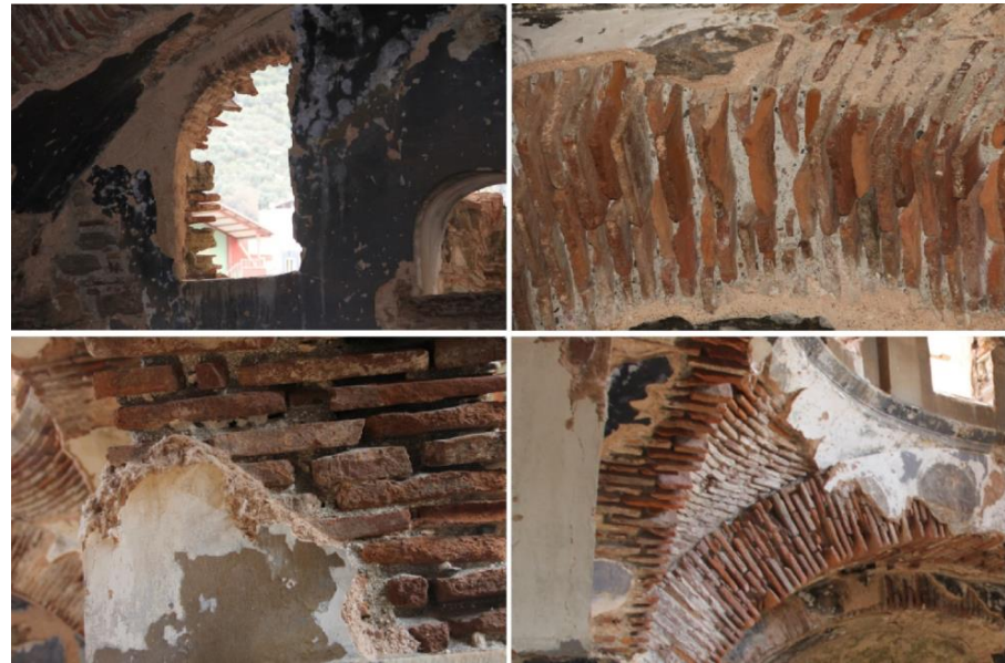
Figure 8. Damages and mortar losses in brick elements.
