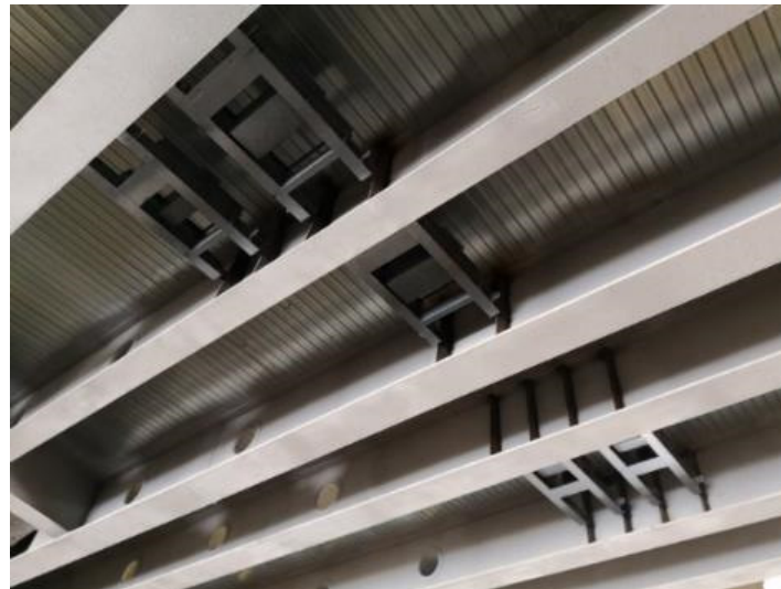
Figure 17. TMDs installed on-site.
