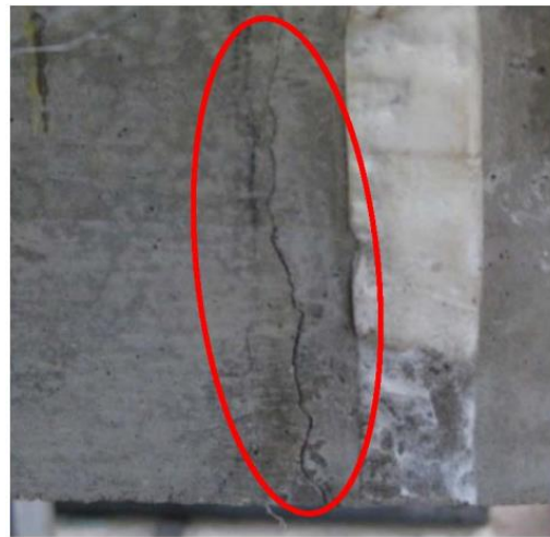
Figure 5. Crack at segmental joints of girders B2 to B4.
