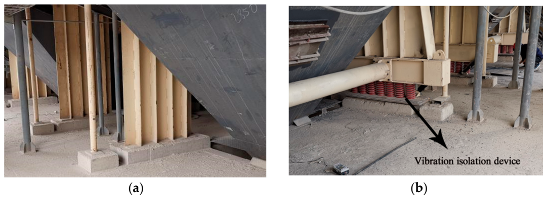
Figure 14. The field arrangement of vibration isolation. (a) Before. (b) After.
