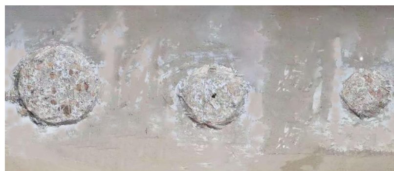
Figure 9. Damages on pipeline.
