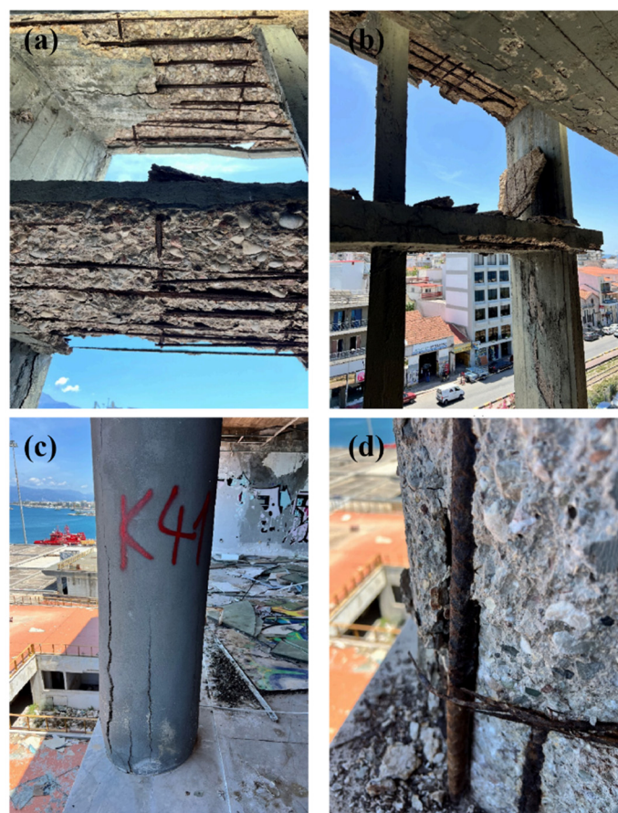
Figure 1. The corrosion and deterioration of reinforced concrete buildings exposed to a marine environment. (a,b) Extensive concrete deterioration requiring major structural intervention; (c) column before concrete removal works; and (d) column after concrete removal works. Reprinted from Ref. [26].
