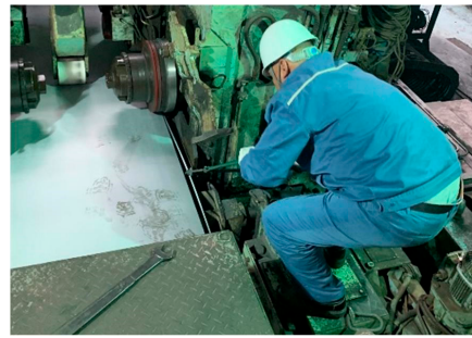
Figure 2. Manual handling of side scrap blockage failure.
