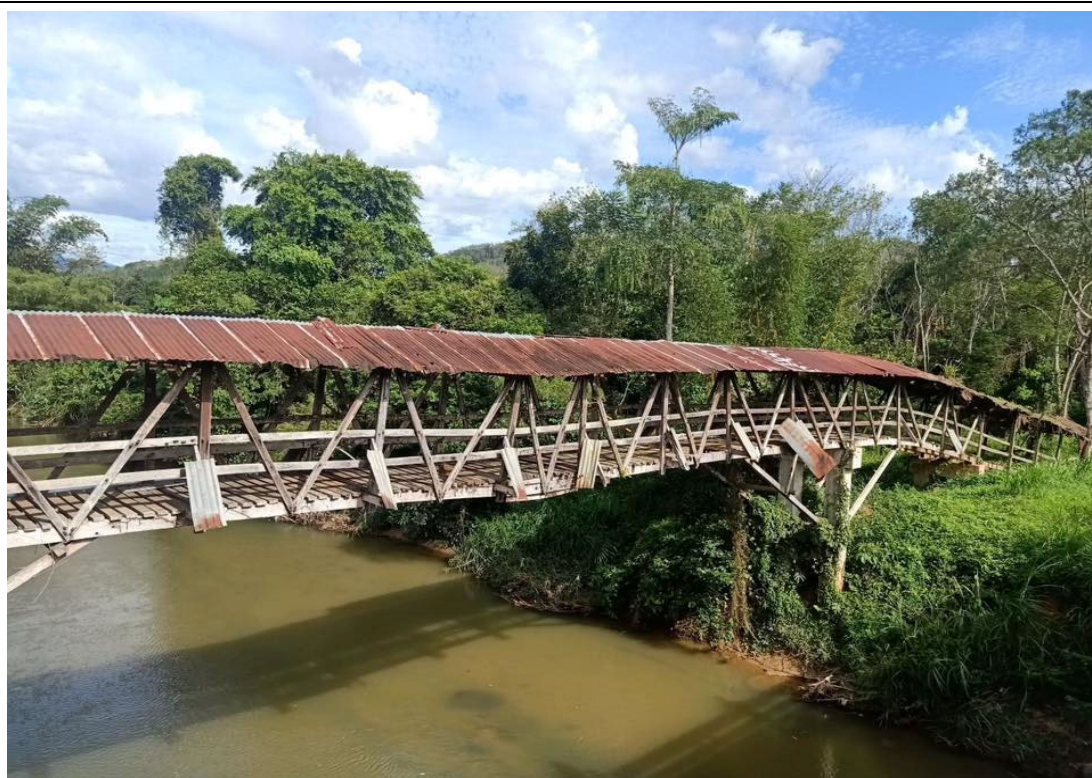
(a) The old Ban Wang Bridge: a cultural asset beginning to deteriorate
