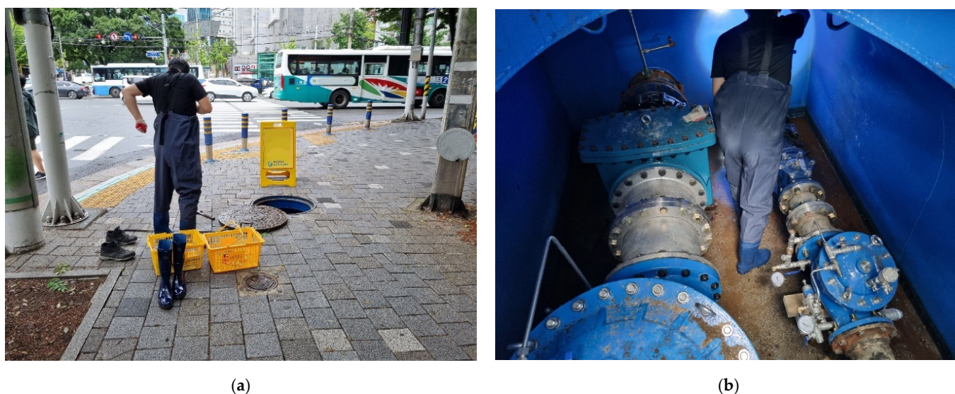
Figure 11. Field investigation of a pressure reducing valve (PRV) chamber at a high-potential site: (a) access and inlet location of the valve chamber; (b) interior layout showing limited available space for additional equipment installation.
