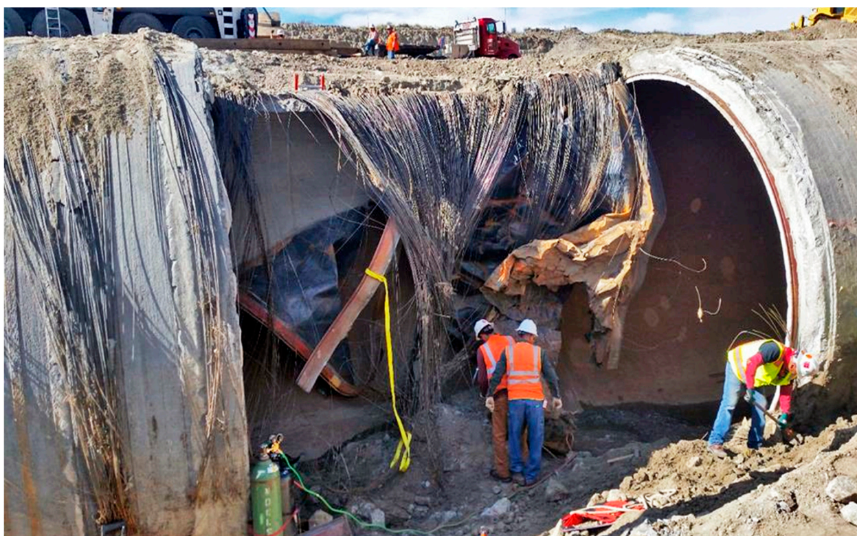
Figure 2. Failed 5.33 m (210 inch) Prestressed Concrete Cylinder Pipe (Photo Courtesy of C. Duke).
