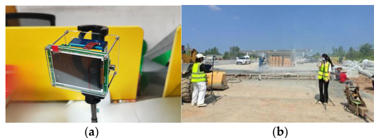
Figure 2. \text{PM}_{10} monitoring equipment and field monitoring setup. (a) \text{PM}_{10} concentration detector used in the field experiment. (b) Layout of monitoring points at the construction site.
