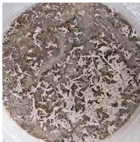
Figure 7. Surface white crystalline deposits from efflorescence on KSCs.
