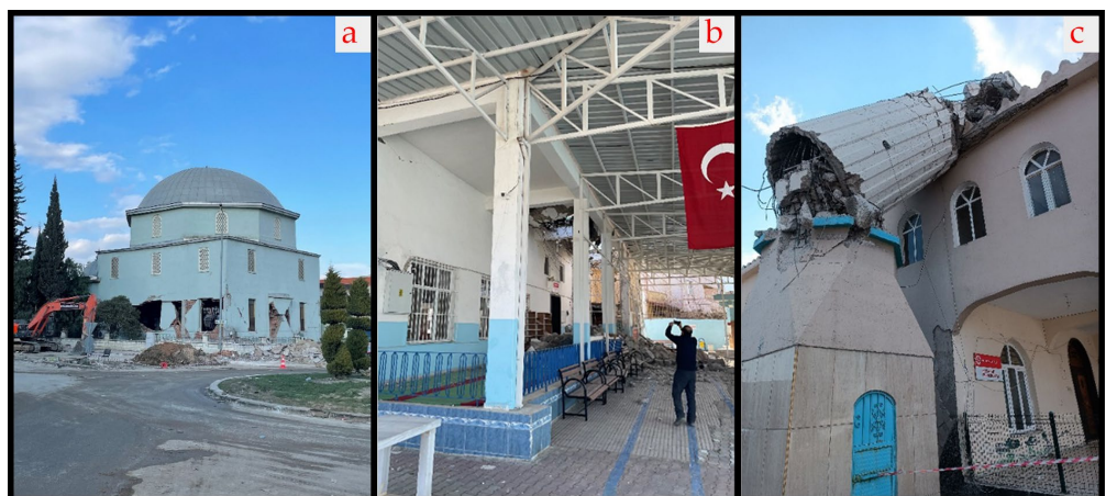
Figure 14. Various types of damage in the RC mosque and minaret structures (a) shear cracks in the infill walls; (b) slab collapse; (c) minaret collapse.
