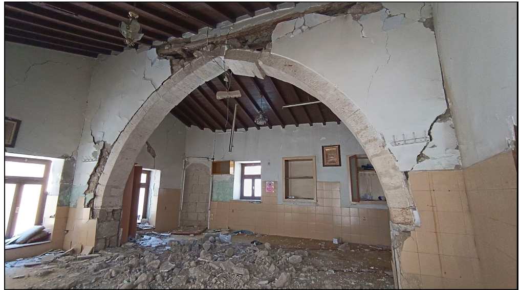
Figure 12. Keystone damage in Debruz Mosque.
