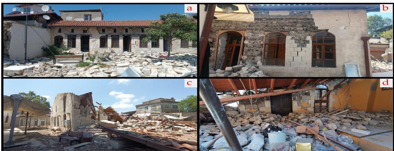
Figure 11. Load-Bearing masonry walls damages: (a) Inadequate Interlayer Bonding, (b) Closer View of Inadequate Interlayer Bonding, (c) Out-of-Plane Displacement, (d) In-Plane Wall Damage.
