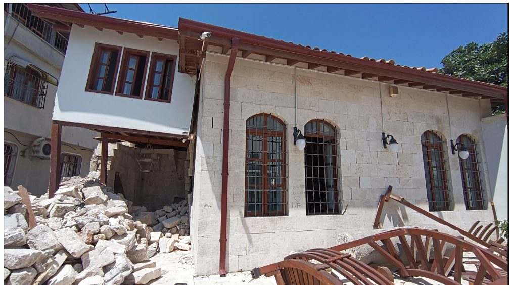
Figure 13. Prevention of collapse performance level due to soft-story (Kürt Fakih Mosque).
