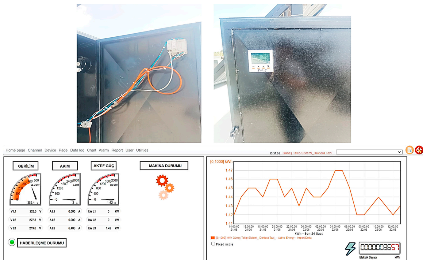
Figure 7. Energy Scada Connection, Visual and Screenshot of Energy Scada software.
