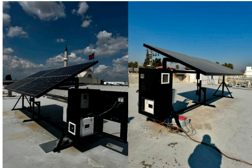
Figure 8. General view of the system installed at Kivanc Textile.
