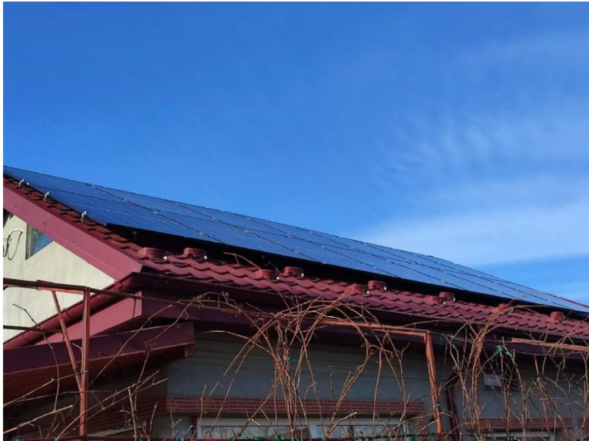
Figure 5. Front view of the PV system.
