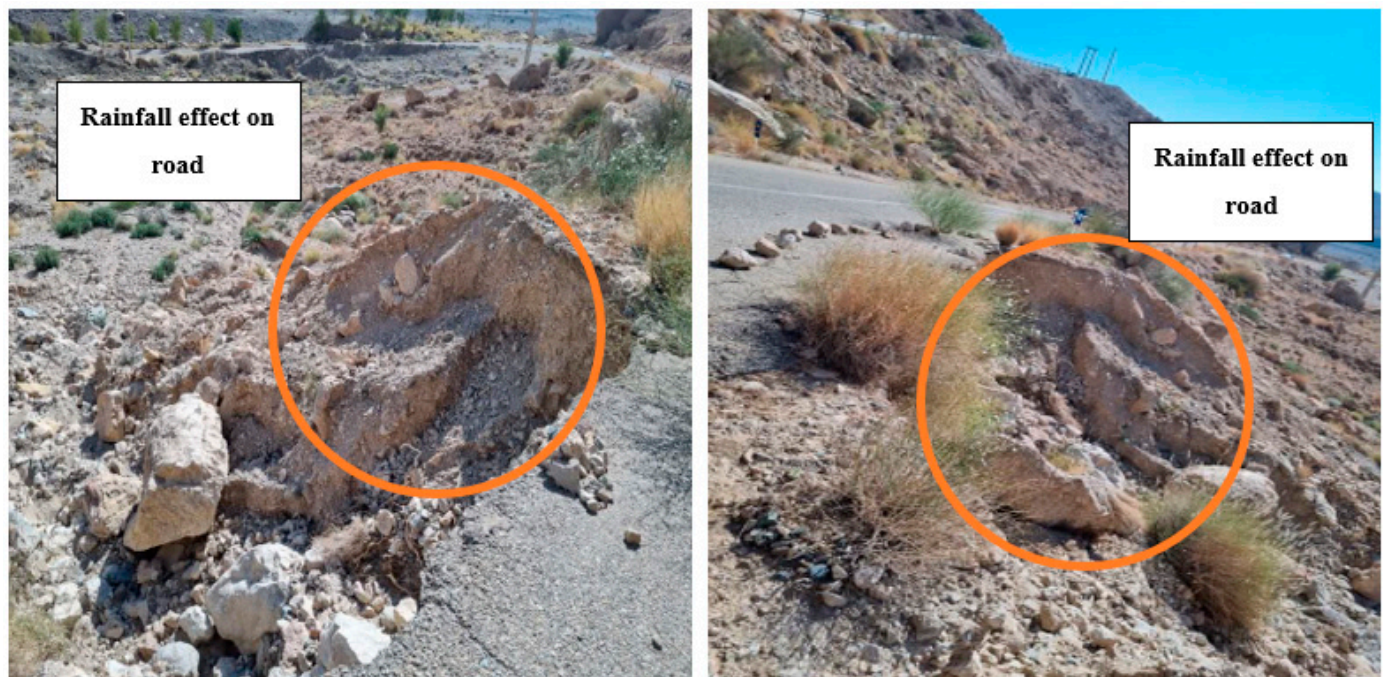
Figure 3. Impact of seasonal rainfall on road stability, shown from the left and right perspectives of the same section of the road.
