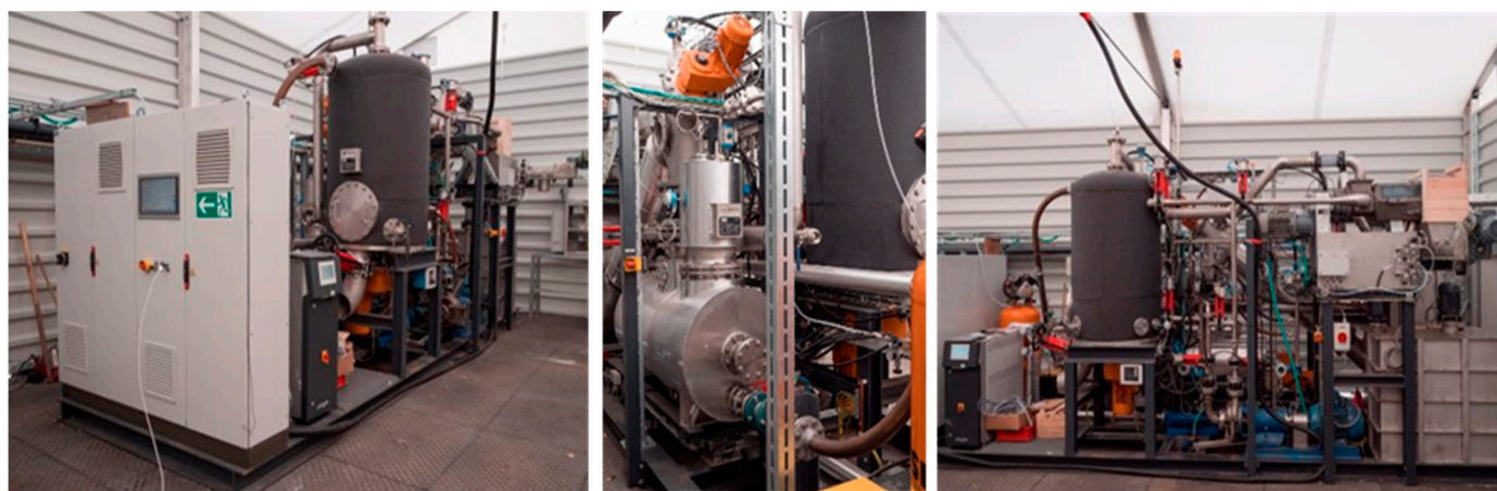
Figure 1. Control cabinet of the TPH system (left), 200 L hydrolysis reactor (center), 400 L expansion tank and pulper, deflaker (right).
