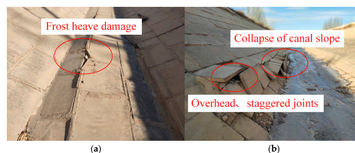
Figure 2. Typical frost-heave damage of concrete-lined canals. (a) Frost-heave damage; (b) collapse, overhead, and staggered joints.
