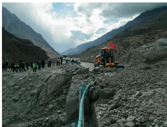
Figure 10. Laqi Gully debris flow site conditions.
