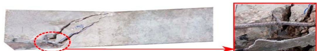
(h) Shear failure and concrete cover separation of a beam (B8)
