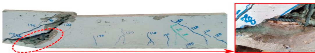
(c) Shear failure and end peeling of a beam (B3)
