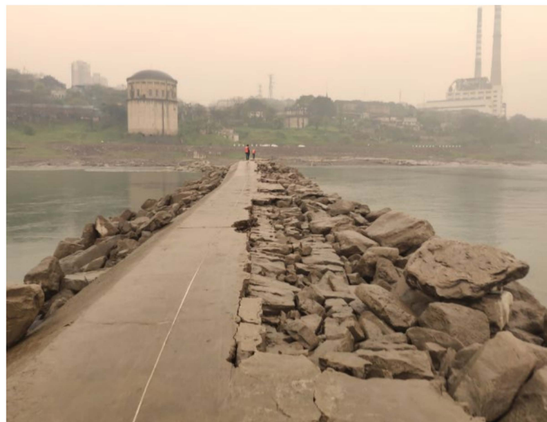
Figure 7. Image from the 2021 site inspection of the Tiemenkan, which showed that most of the dam surface has been half-stripped (the photo is from the daily shooting data of the Changjiang Waterway Bureau of China).
