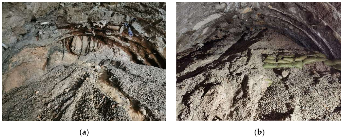
Figure 5. Water and sand gushing from fierce sanding dolomite in Xiaopu 2# construction adit. (a) Xiaopu 2# adit's fierce sanding dolomite with water gushing. (b) Xiaopu 2# adit's fierce sanding dolomite with sand gushing.
