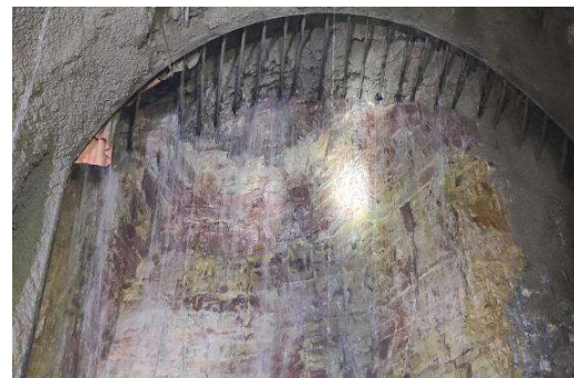
Figure 4. Intense sanding dolomite seepage of Xiaopu 2# construction adit.
