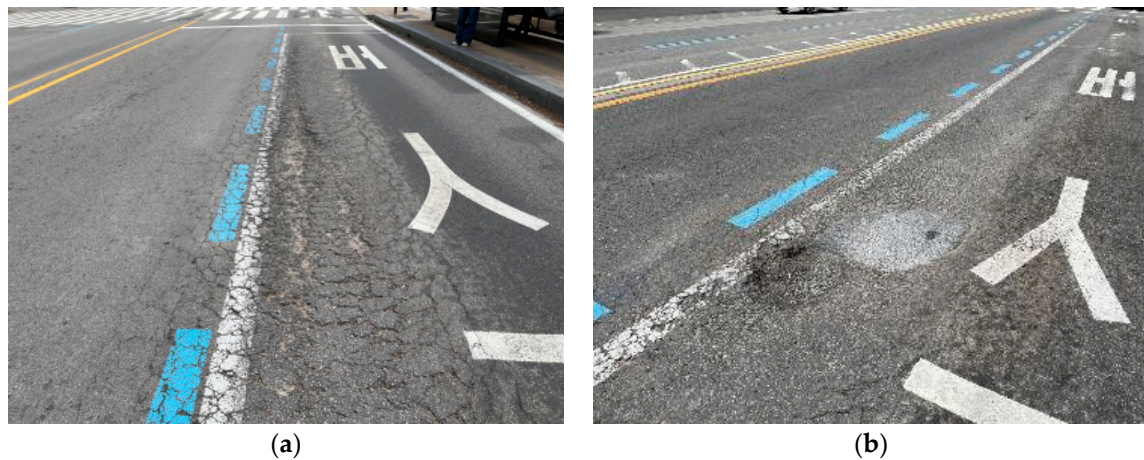
Figure 1. Damages of bus stop asphalt concrete pavement: (a) cracks and rutting; (b) pothole.
