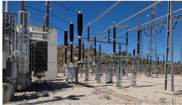
Figure 6. The São Martinho substation in Alto Douro.
