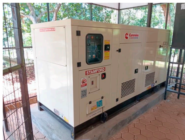
Figure 2. Diesel generator set Cummins 6BTAA5.9-G12.
