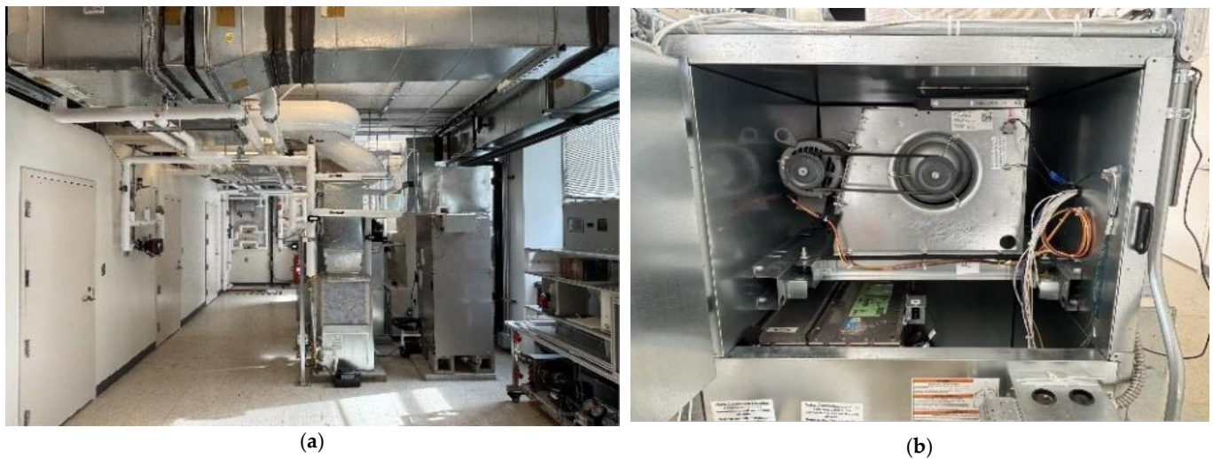
Figure 1. BEAST laboratory facility and tested equipment. (a) BEAST HVAC laboratory. (b) Tested air handling unit.
